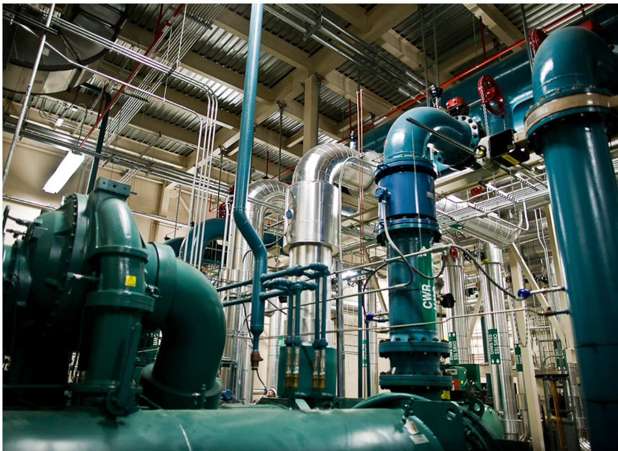
ChemCal Water Treatment at the JJ Pickle Research Facility in Austin, TX
